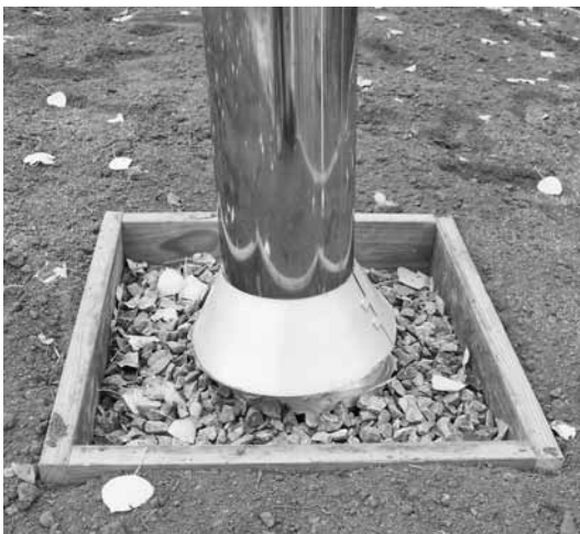
Fig. 8.12: Drainage is the better part of waterproofing! Any projection through the membrane is a potential leak. I boxed around the stovepipe with pressure-treated 1-by-6 material and placed crushed stone over the Enkadrain®. Water is quickly carried away to the edge of the building.
