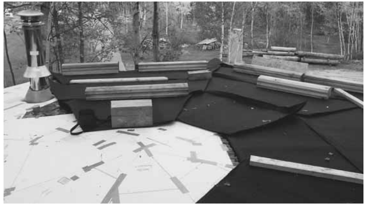
Fig. 8.7 (left): Installing a woodstove chimney. Any projection cut through the membrane has to be treated very carefully, with both waterproofing and drainage. As our Metalbestos® stovepipe has an 8" outside diameter, we made a hole of 12" in diameter through the Bituthene®-covered planking. A reciprocating saw works well for cutting the hole. This way, the chimney has the required 2" clearance from combustible material. The Roof Support Package (Metalbestos® part RSP) unit shown has two adjustable metal flanges which can be screwed to the planking, allowing the installer to plumb the stovepipe itself to a true vertical.
