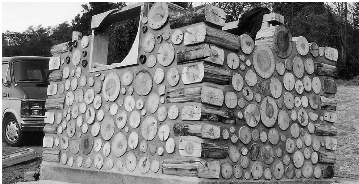
1.9. This small pump-house in North Carolina was made with single-wide quoins, cut from tulip poplar with a chainsaw, then water-sealed to minimize water absorption from mortar to wood. The staggered length of the quoins is clear in this image.
