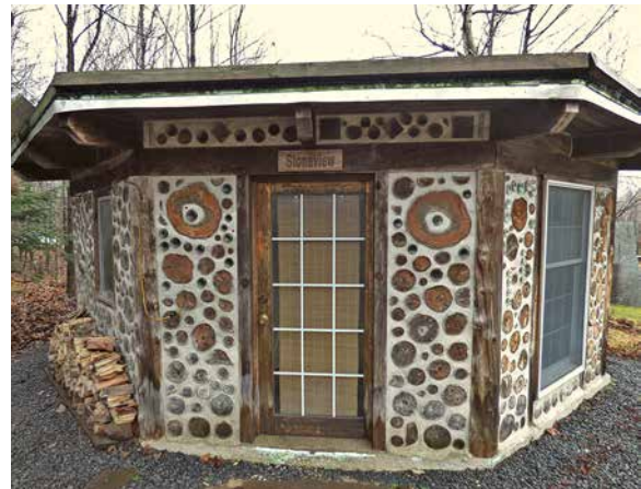
1.16. Stoneview is an octagonal guesthouse with eight 8-inch by 8-inch girts joined over eight special posts. Both the door jambs and the long window frames (all 4-inch by 8-inch stock) extend from the floating slab to the underside of the girts. Full framing details are in my book Stoneview: How to Build an Eco-friendly Little Guesthouse (New Society Publishers, 2008.)
