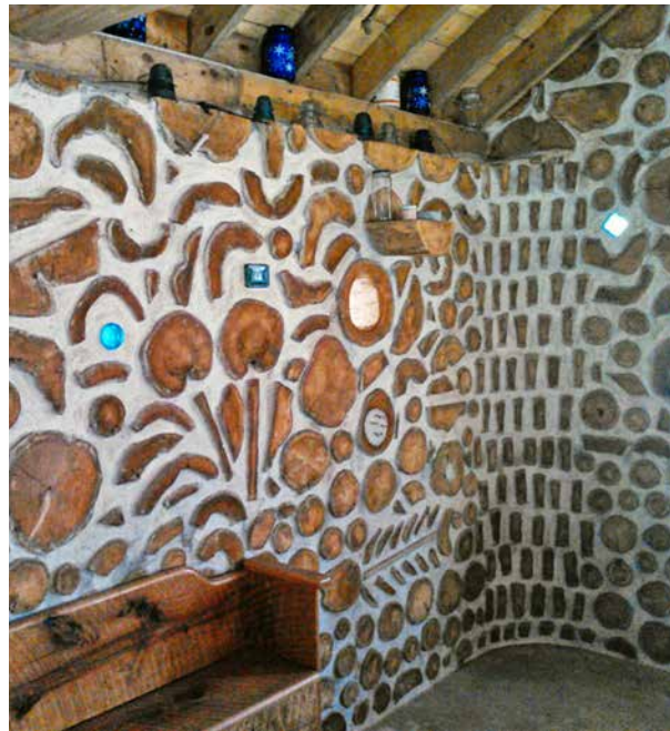
1.18. Interior of Bull Nose Cabin. Note that the corner logs have all been tapered. Credit: Lonnie Sobeck.
